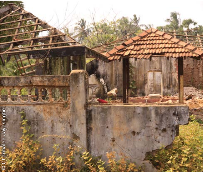
Damaged house in Mullaitivu district. One of the issues to solve in the reconstruction was land tenure, as many families had lost their titles during the conflict.
