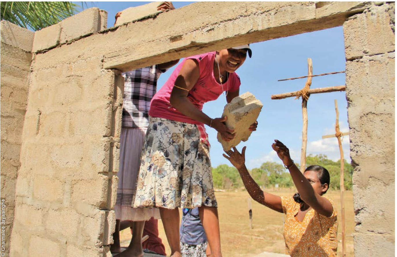
Women engaged in construction training, Kilinochchi district. Gender mainstreaming was promoted through the mandatory representation of women in reconstruction committees, as well as involving women in capacity-building and construction activities.
