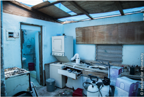
Many houses reported damage to roofing, as well as to indoor spaces. Beyond the building envelope, when possible, the project also supported households to repair kitchens and bathrooms.
