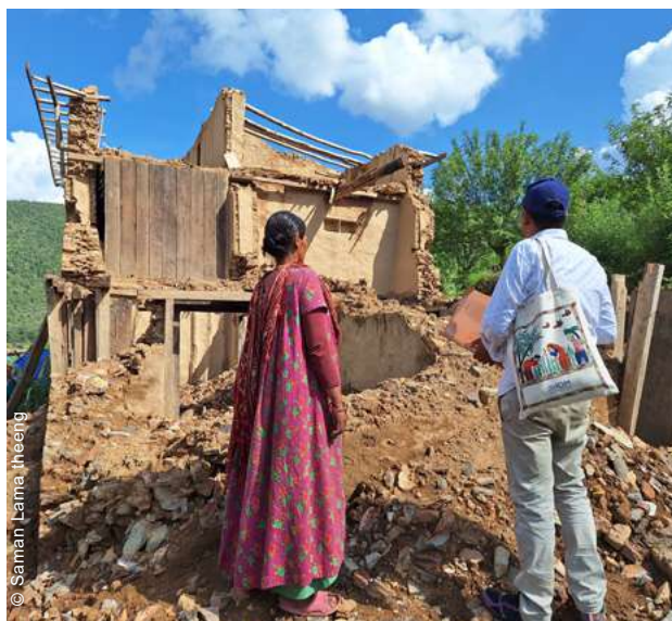
A community member stands amid the ruins of her home during a post-earthquake assessment, in Nepal.
