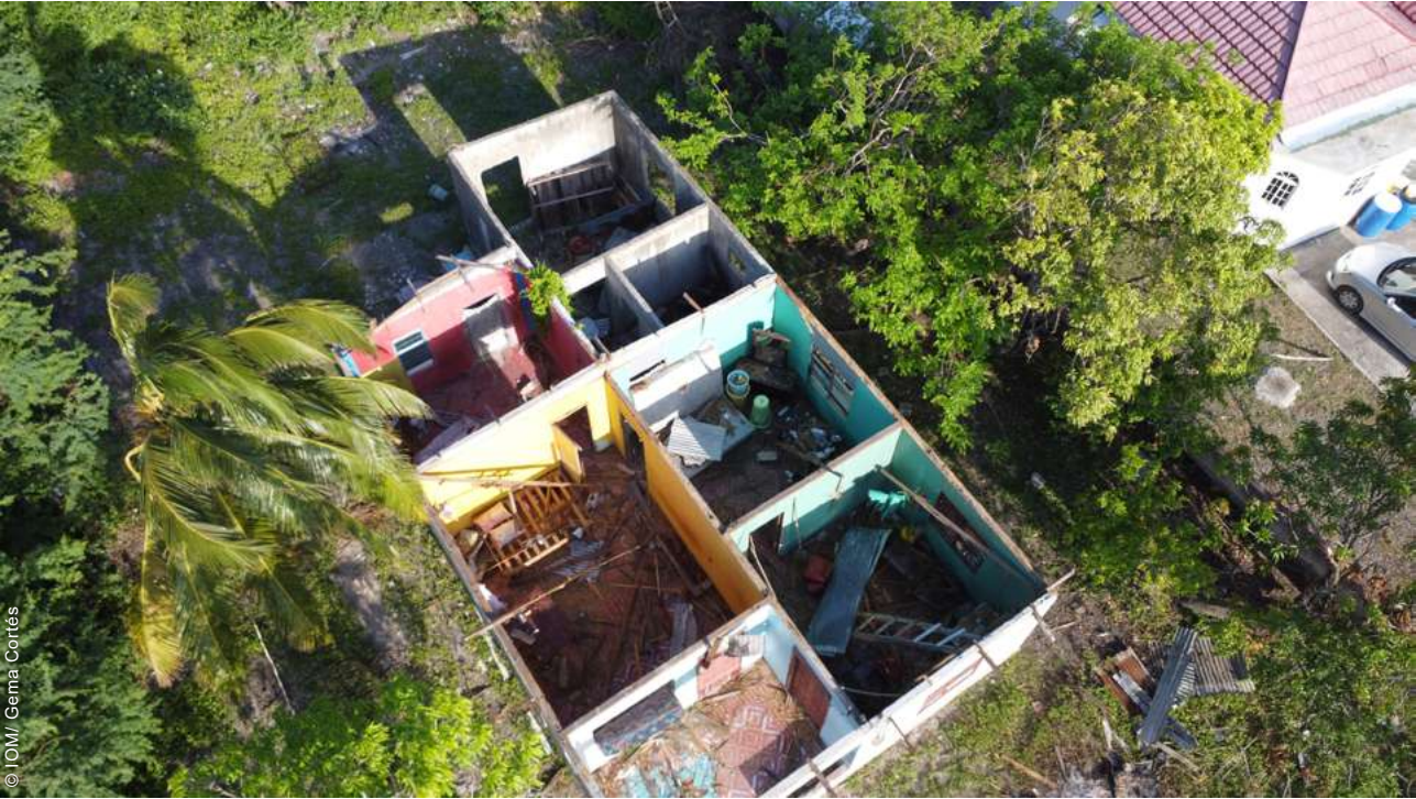
An aerial shot captures the devastation left by Hurricane Beryl, showing a roofless house in Jamaica. The powerful storm caused widespread destruction, leaving many homes and buildings severely damaged and communities struggling to recover.
