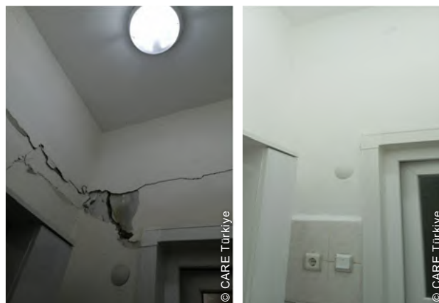
Following the earthquake in 2023, some of the activities were adapted.
