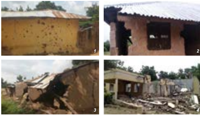
Damage was categorized in four groups. 1) Bullet holes on the external walls but not penetrated inside; hairline cracks in very few walls; fall of small pieces of plaster only. 2) Doors and/or windows need to be replaced, damage to brickwork 10%. 3) Failure of structural elements, damage to walls 25%. 4) Completely damaged with bullet holes, serious failure of walls; partial structure failure of roof and floor.
